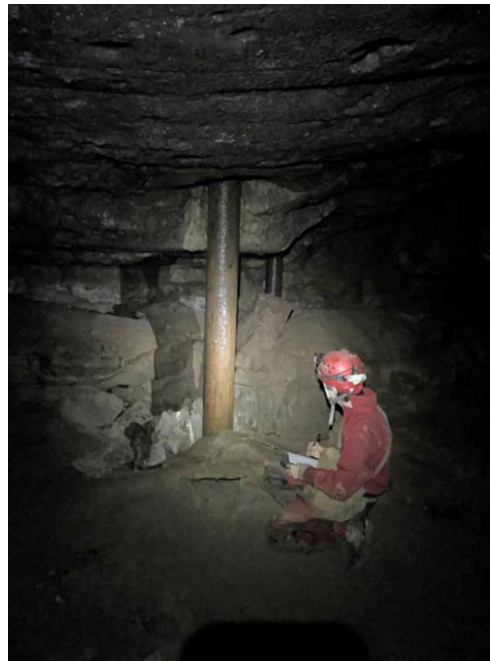
Figure 3. Drainage well casings in the Breakdown Canyon section of Hidden River Cave.
